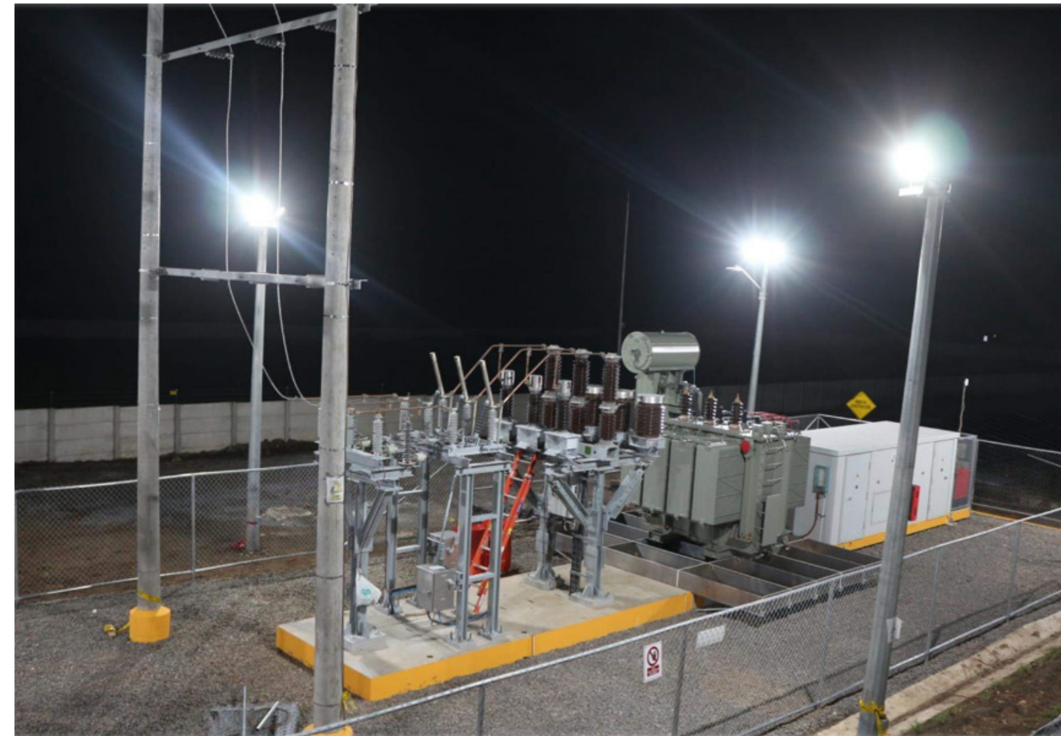
Traditional Outdoor Substation
