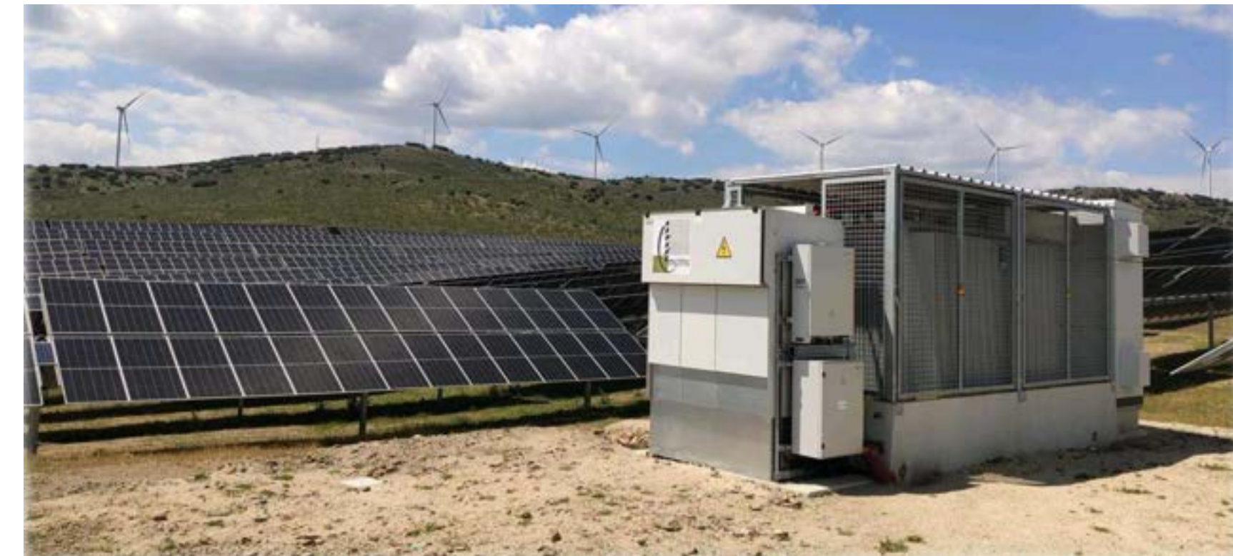
"PV Solana, Spain"
