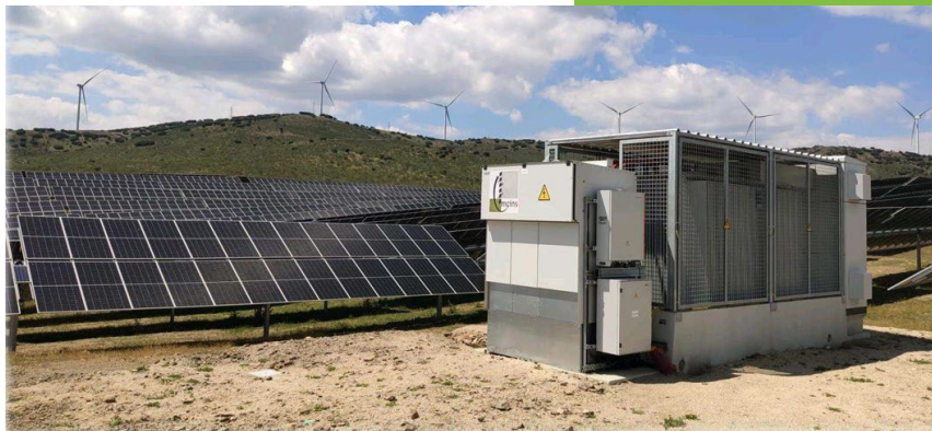
"PV Solana, Spain"
